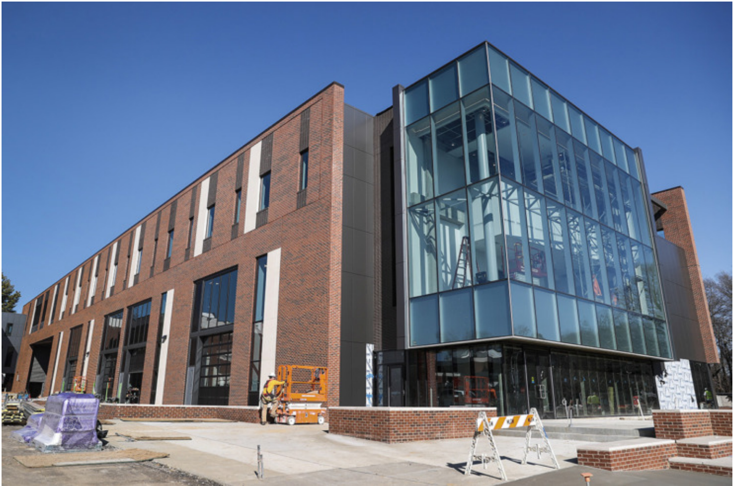
The STEM classroom and research building at the University of Memphis connects to the three-story Herff College of Engineering. (Mark Weber/The Daily Memphian)
