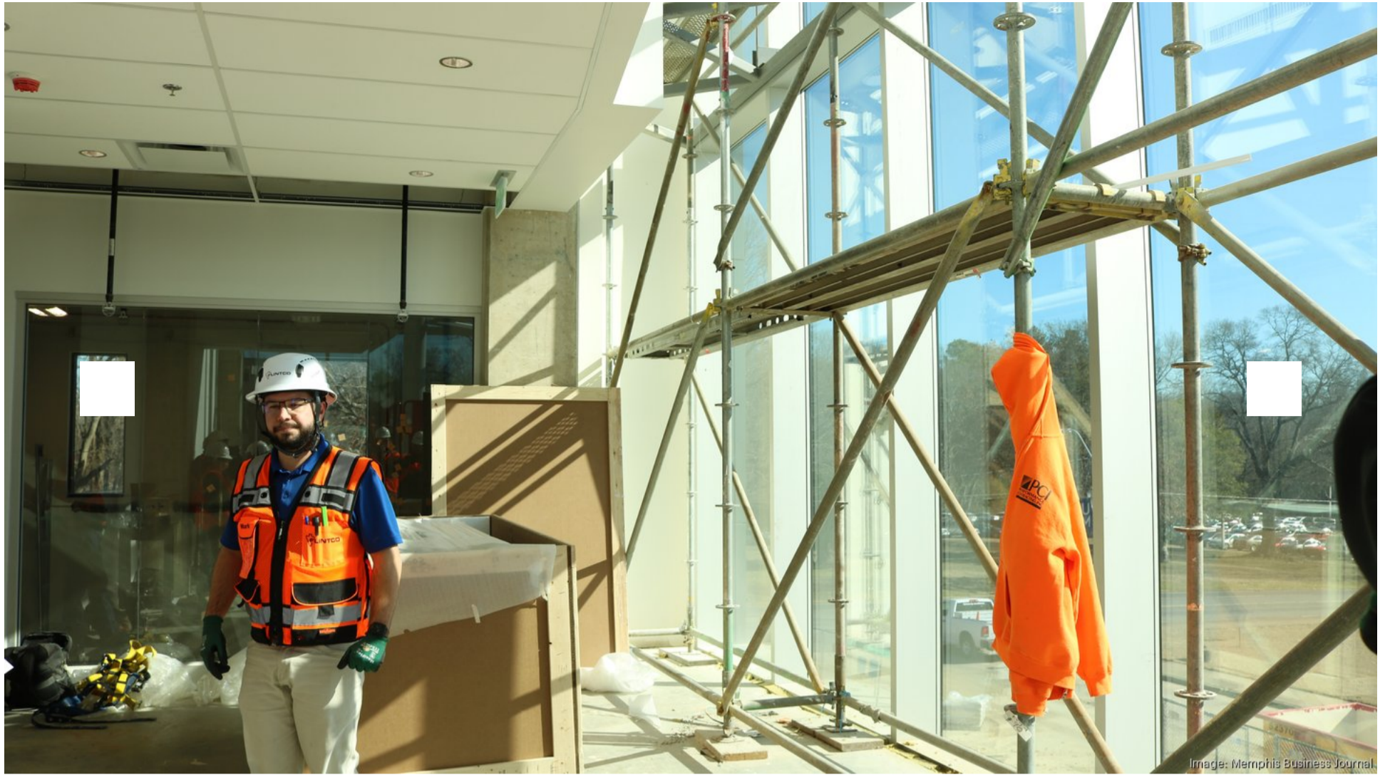
Mark Pasino, project manager at Flintco, guides a tour of the STEM Research and Classroom Building during construction. The building features a glass facade that overlooks the U of M's campus.
